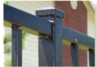
A three-year old painted fence that has already been re-painted four times.
